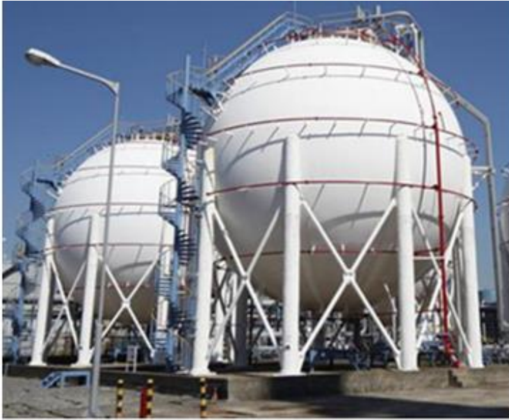
Figure 7: Above ground Spherical LPG pressure storage tank (WEEN Consult Limited, 2020)
