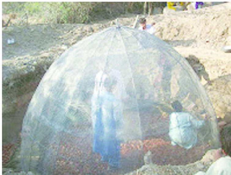
Fig.2. 14 -Ferro-cement biogas plants (Construction of a biogas plant in Mirpurkhas Sindh Pakistan 2012)
