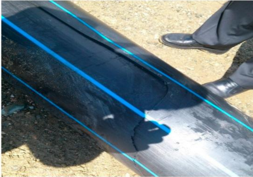
Figure 20. Brittle crack of pipe (photo Scarlatescu).
