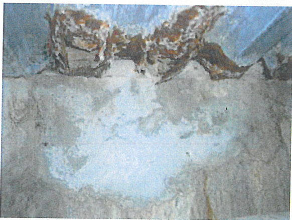
Figure 1-4 Corrosion of galvanized fluted steel floor deck. The floor is at grade level. The source of the water is rainwater seepage.
