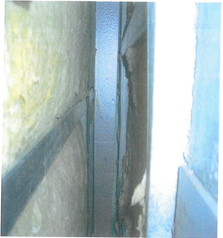
Condensation occurs on a C-channel at the top of a parapet wall located in a cold climate. The building is humidified and pressurized with filtered outdoor air to maintain specified interior conditions.
