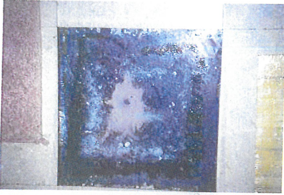
Figure 1-13 Tile adhesive that failed to cure because of water in the concrete and high pH. The tile can be removed by hand. The floor is a concrete slab-on-grade. The water visible in the photo evaporates into the room after several minutes. Its source may be liquid water wicking up from the sub-slab fill or water vapor migrating through the slab.
