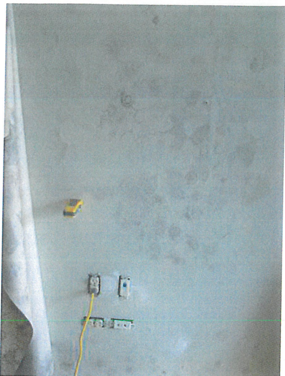
Figure 1-7 Condensation behind vinyl wallpaper in a warm, humid climate. Condensation and mold growth occurs behind the vinyl wallpaper on both exterior and interior walls. Air leaks in the return plenum of the air handler depressurizes the interior and exterior wall cavities. Warm, humid exterior air is drawn from outside through air leaks in a heavy masonry wall.
