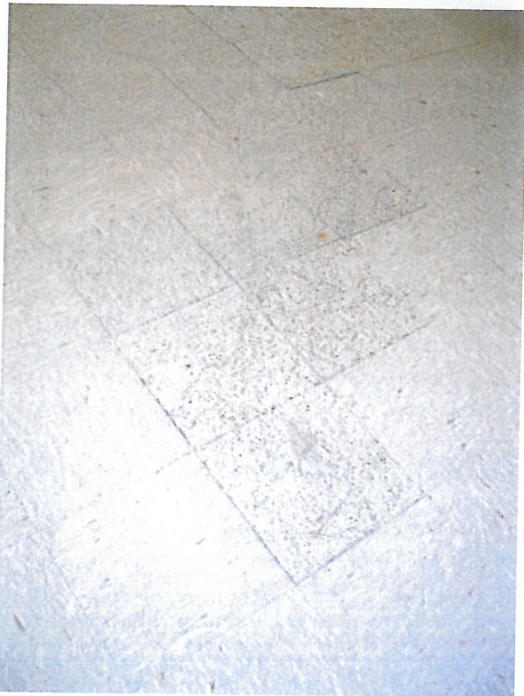
Figure 1-3 Mold growth on vinyl floor tile. Long-term high humidity provided moisture that was absorbed into the cool vinyl tile and supported mold growth. Also note that the high humidity caused the adhesive attaching the tile to the floor to fail, allowing the tile to become loose.
