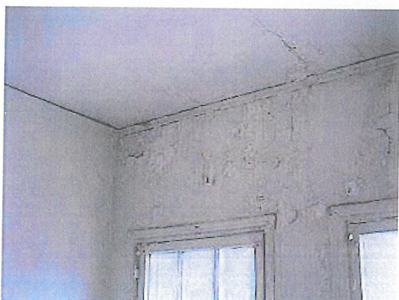
Figure 1-8 Rainwater leaks in a rooftop parapet wall result in damaged plaster and peeling paint. Rainwater is drawn into this brick assembly by capillary action, and the moisture is aided in its downward migration by gravity. The peeling paint contains lead and results in an environmental hazard as well as physical damage to the plaster.
