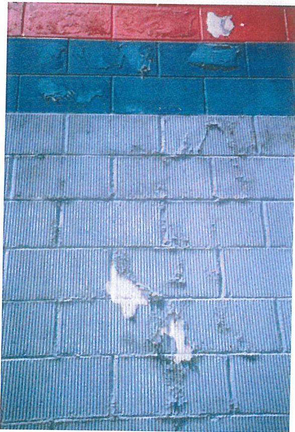
Figure 1-6 Blistering paint on split face concrete block. Wind-driven rain is the source of moisture contributing to the damage. Water wicks into the concrete masonry unit (CMU) through pin holes in the paint. The sun drives water vapor through the CMU. The assembly cannot dry to the interior because low-vapor-permeability foam board, taped at the joints, insulates the interior surface of the wall. The wall remains saturated throughout the spring, summer and fall. The same paint on areas of the wall sheltered from sun and rain shows no damage.
