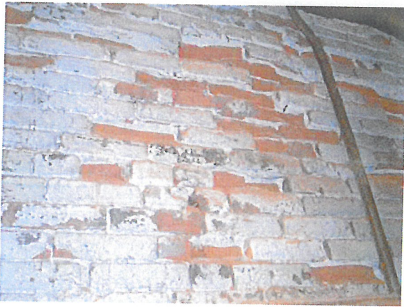
Figure 1-14 Damage to bricks caused by the migration of soluble salt through them. Salts in the brick or mortar dissolve in rainwater that wicks through the brick. The water evaporates in the building's interior, and the salt left behind crystallizes and splits the surface layer off the brick, exposing its interior. This process is called sub-fluorescence.
