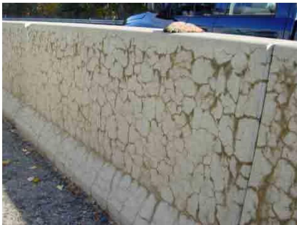
Figure 2 Cracks in concrete due to ASR
