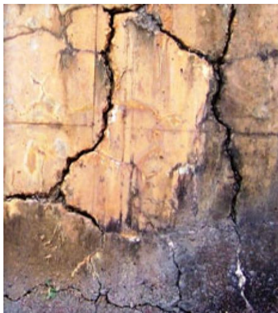
Figure 1 Cracks in concrete due to ACR
