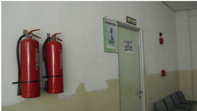
Fig. 12 Fire resistance equipment. Picture Source Adamy (2014)
