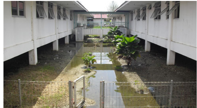
Fig. 11 Water stagnant and debris under the semi stilts buildings Picture source Adamy (2014)
