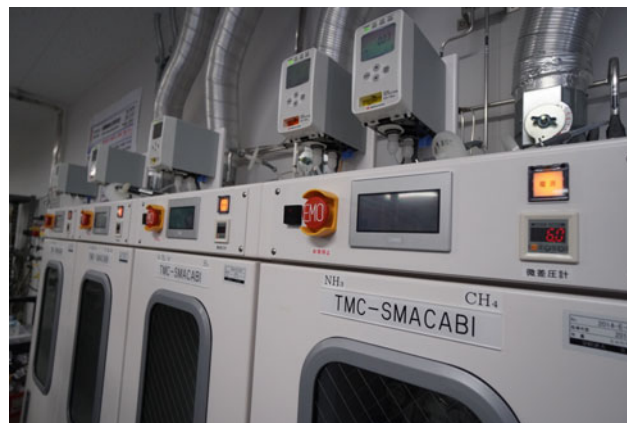
Fig. 4 Toxic and flammable gas monitoring system
