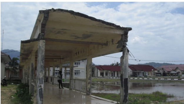
Fig. 10 Damaged corridors. Picture Source Adamy (2014)
