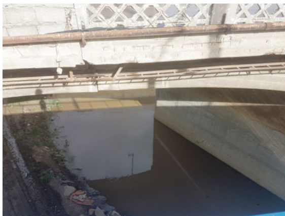
Fig. 8 Pictures view of the waters of Oude El Harrach from the ring road bridge
