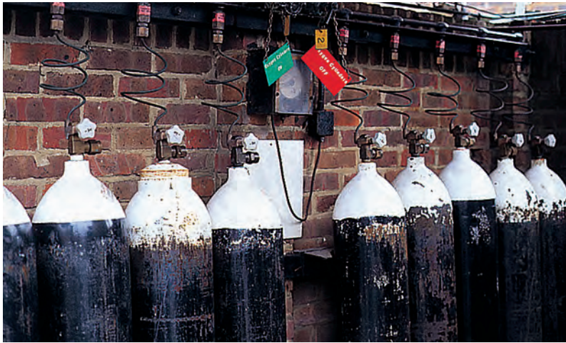
Fig. 1.17 An oxygen cylinder manifold.
