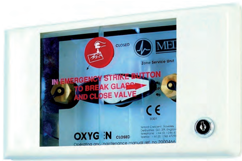
Fig. 1.15 An Area Valve Service Unit (AVSU).
