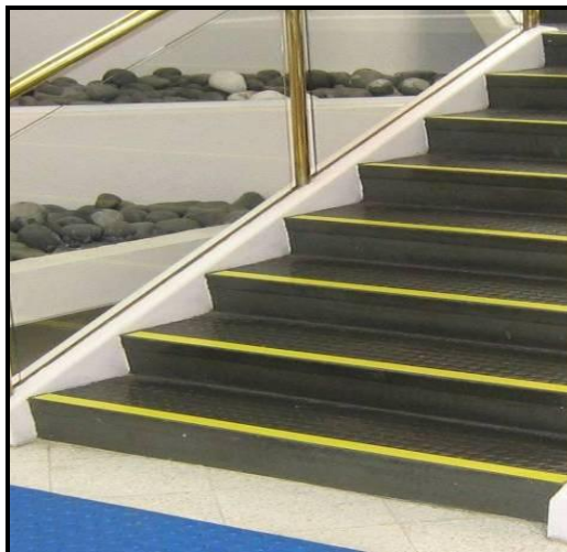
Photo 1 shows a set of stairs with no open risers
