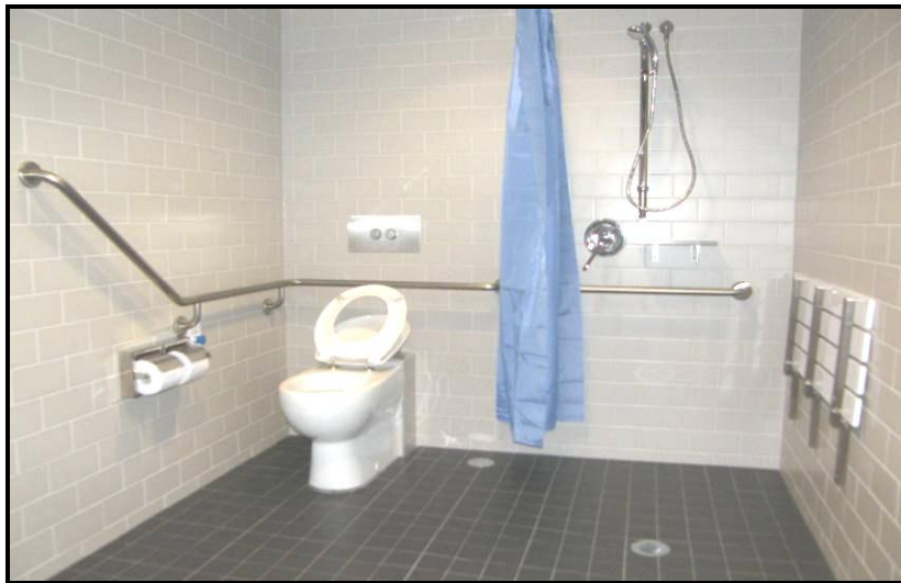
Photo 1 shows a good example of correct installation of toilet and shower fittings
