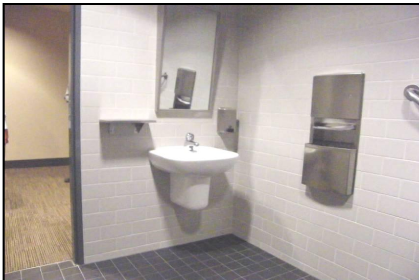
Photo 2 shows a good example of the installation of a washbasin and other fittings, including a shelf as required by Table F2.4 of the BCA, note that tilt mirrors are not a requirement of AS1428.1.
