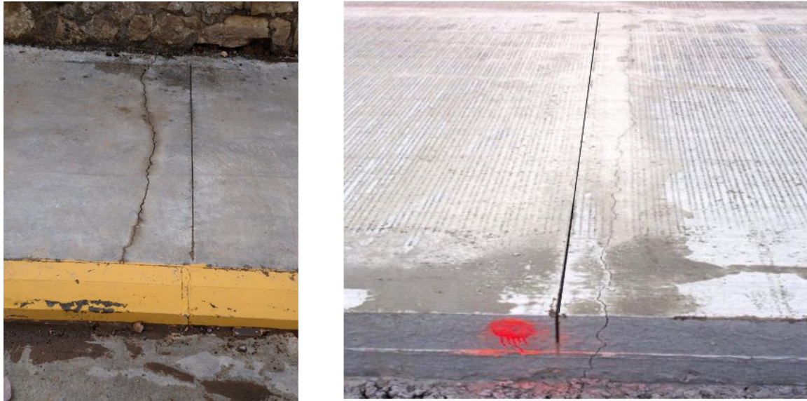
Figure (11): Late Saw Cuts
