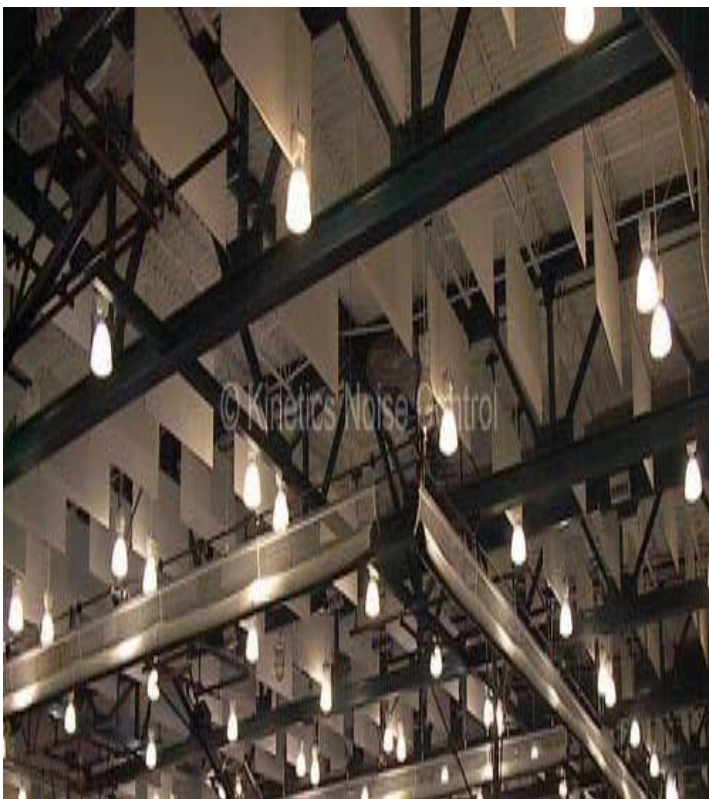
Noise Control Baffles (fiberglass)
