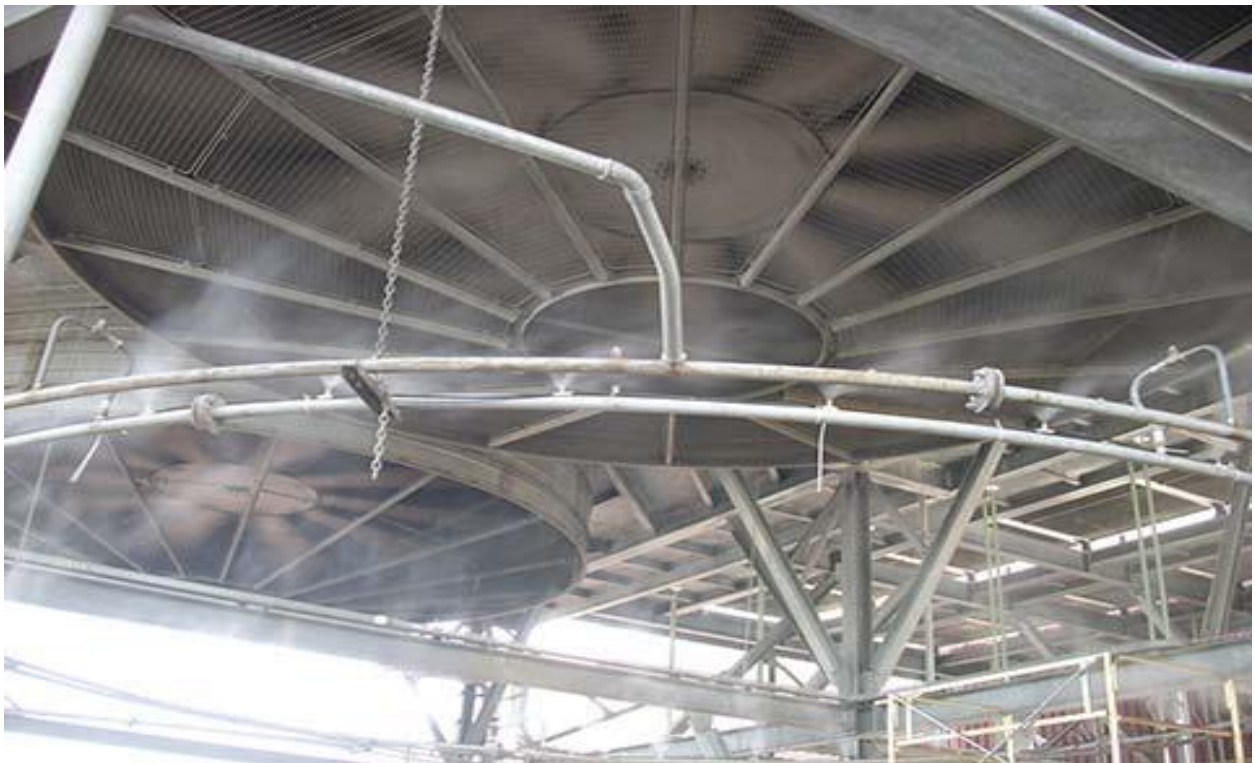
Figure 14- Practical misting system
