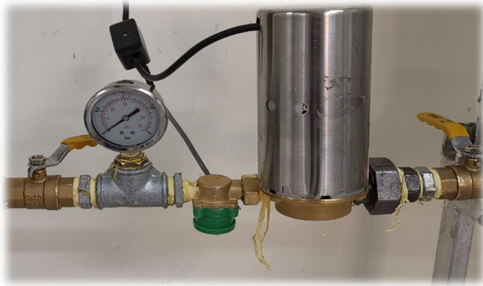
Figure (6) The pressure pump.
