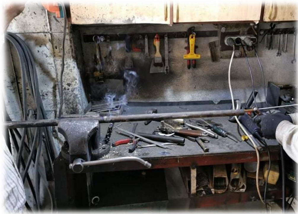
Figure (5) Making crack by welding the length of each crack case have been from 0.01m in case 2 and increased to 0.475m in case 9.
