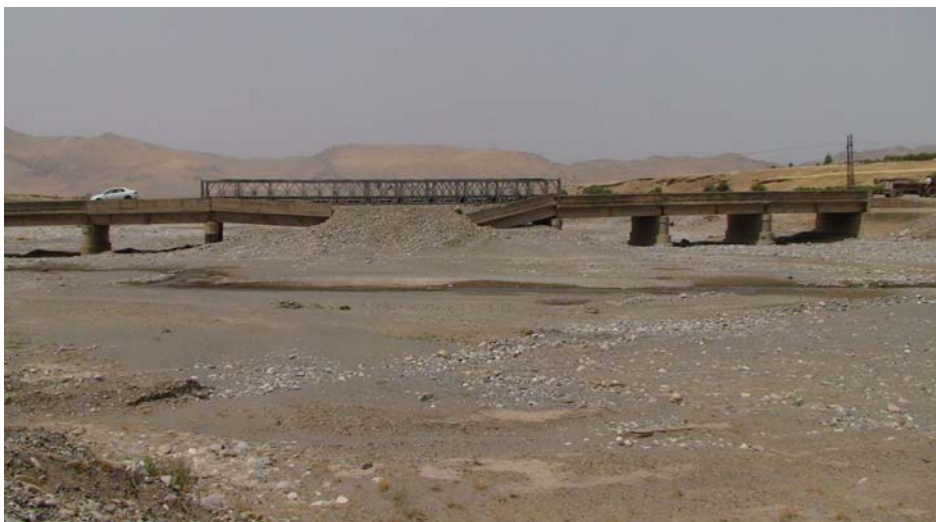
Zharawa damaged bridge
