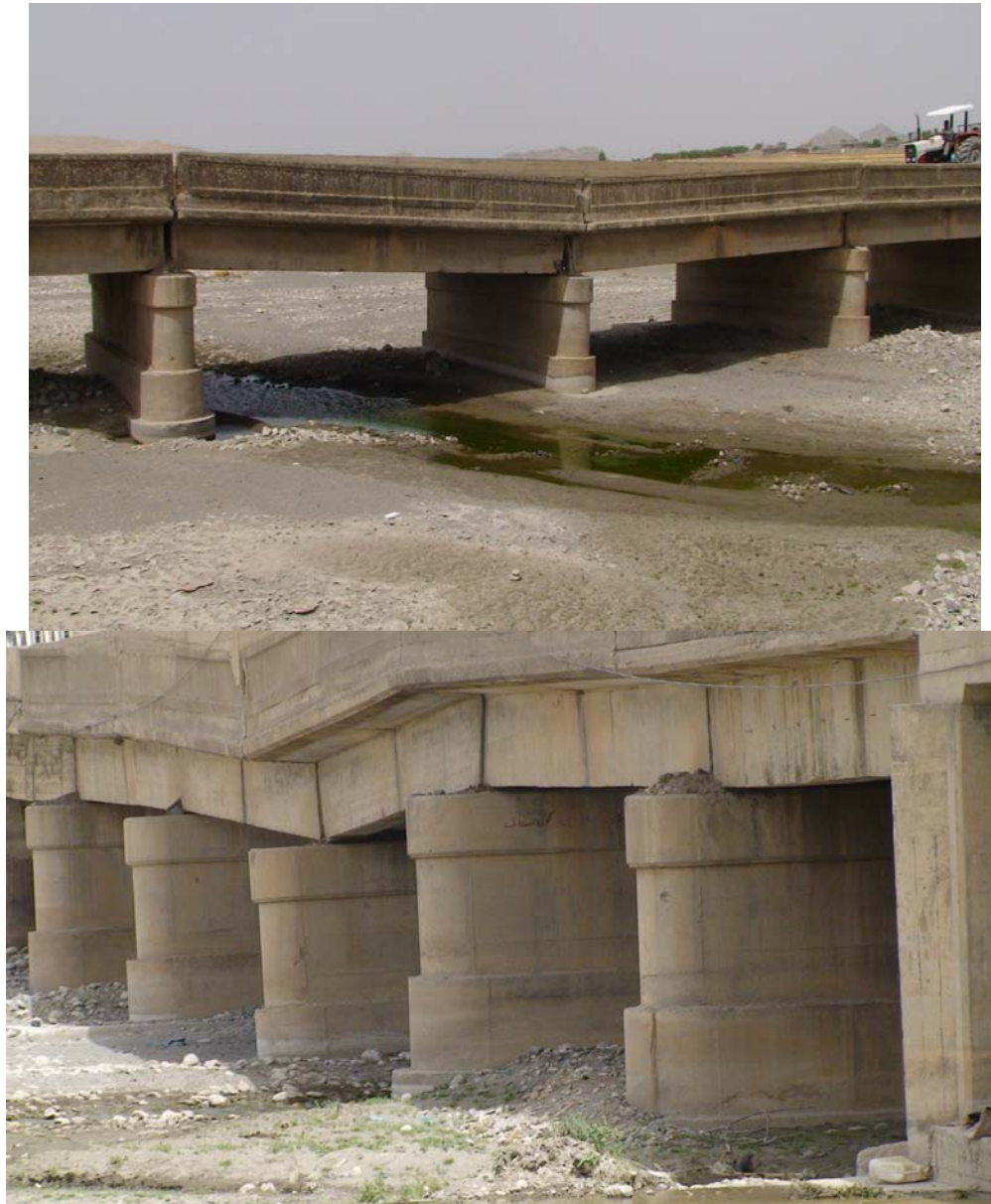
Failure of Zharawa bridge (local scour)
