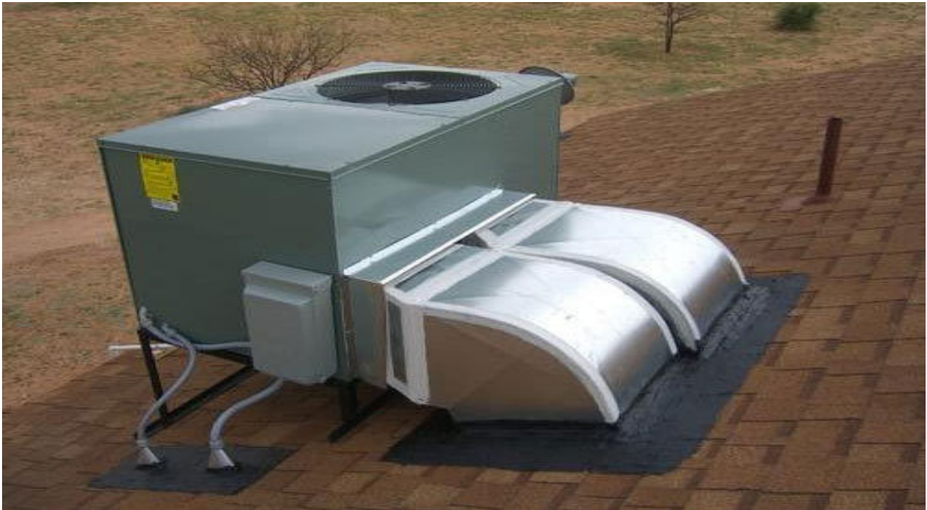
Rooftop package unit (RTU)
