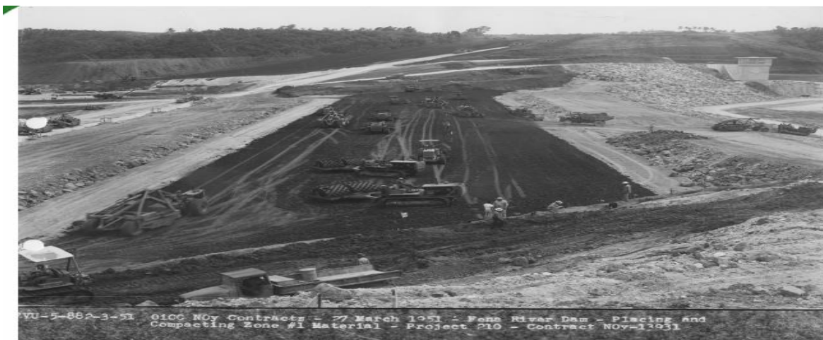
Placement of earthen clay core, up and downstream filters, and rockfill shells at Fena Dam on Guam by Navy Seabees in 1951. Upstream is to the right.
