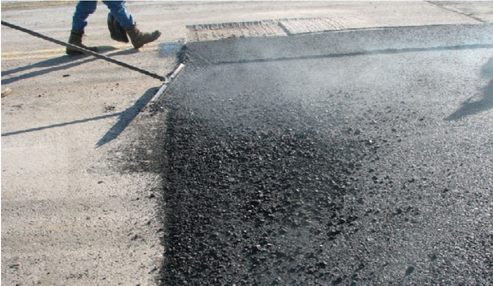
Figure ٢-٣-٢. Poor Raking at Joint
