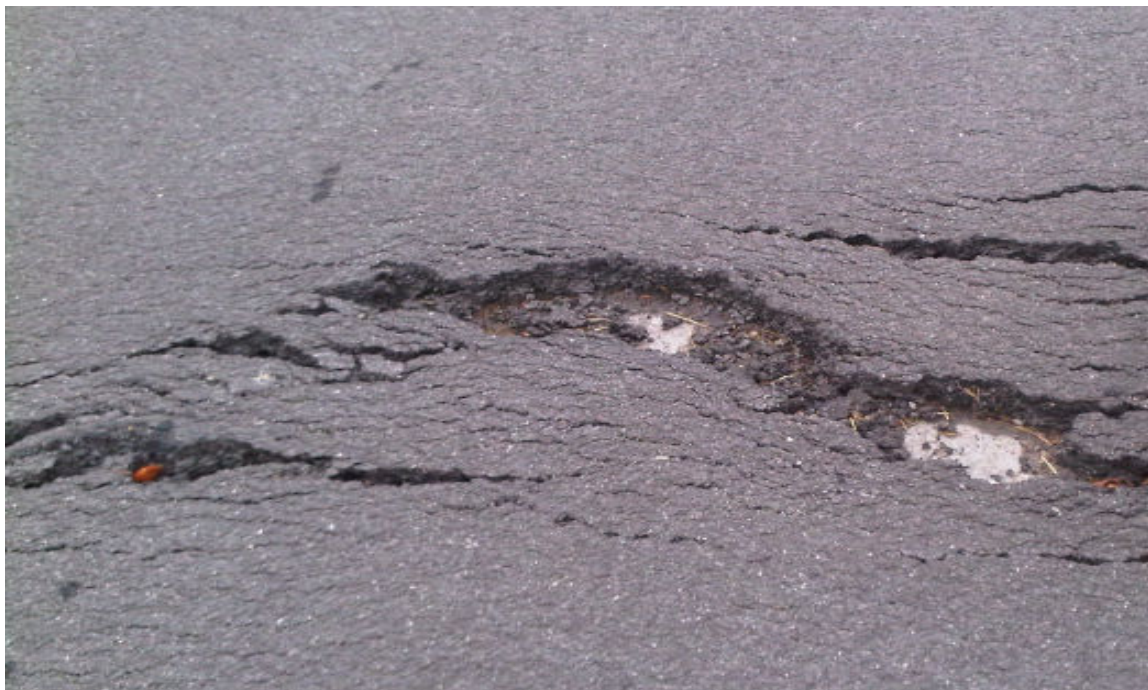
Figure ϣ-ϛ. Tearing of Mat – Center
