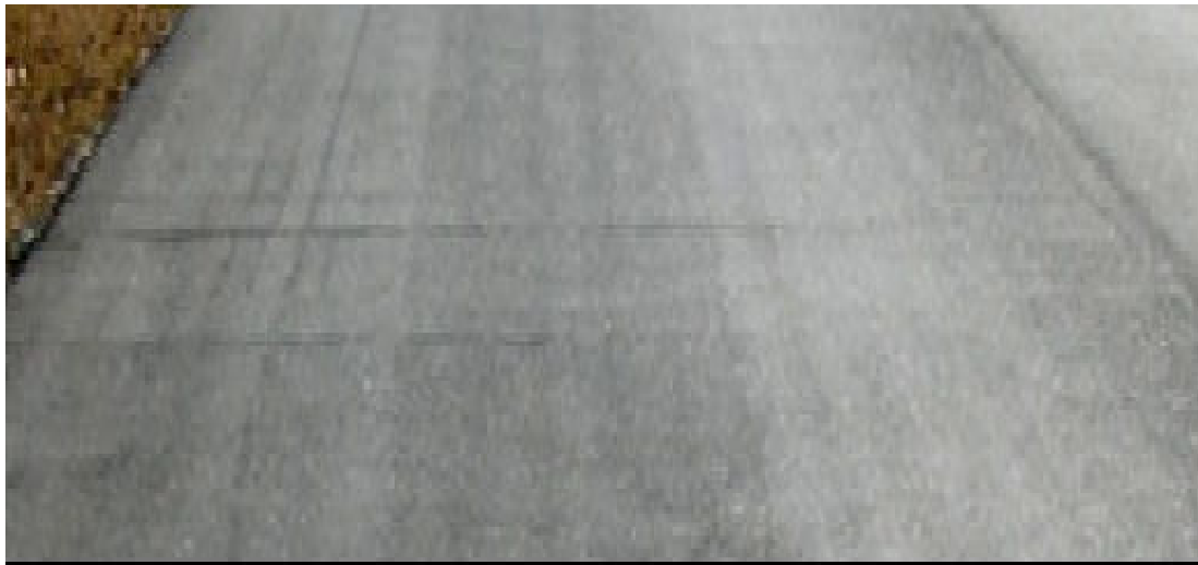
Figure ٢- ٤- ٤. Marks Due to Truck Bumping Paver
