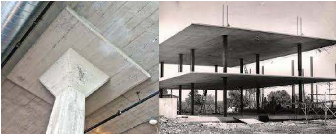
Flat slab with both drop panels Simple flat slab and column heads
