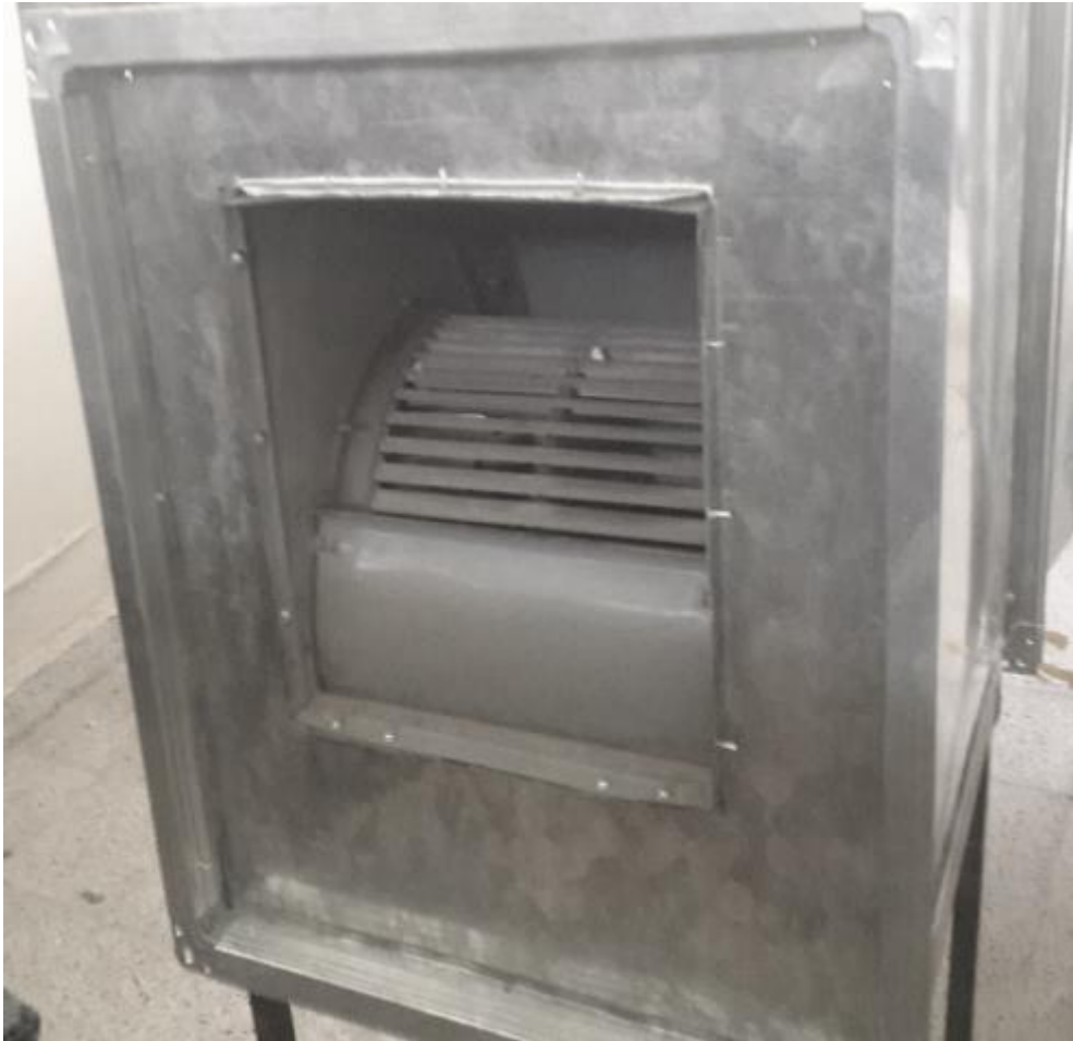
Figure (8) supply fan.
