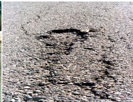
Raveling caused by segregation
