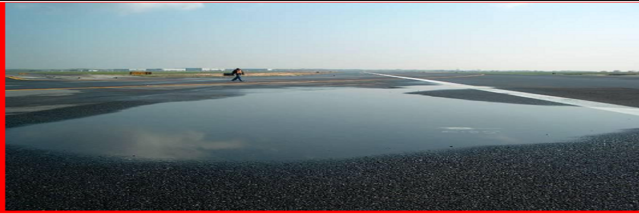
High severity leads to ponding and can cause hydroplaning of aircraft.
