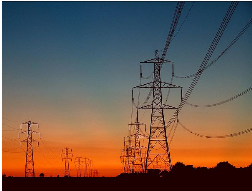
Figure (3) Overhead Power Lines
