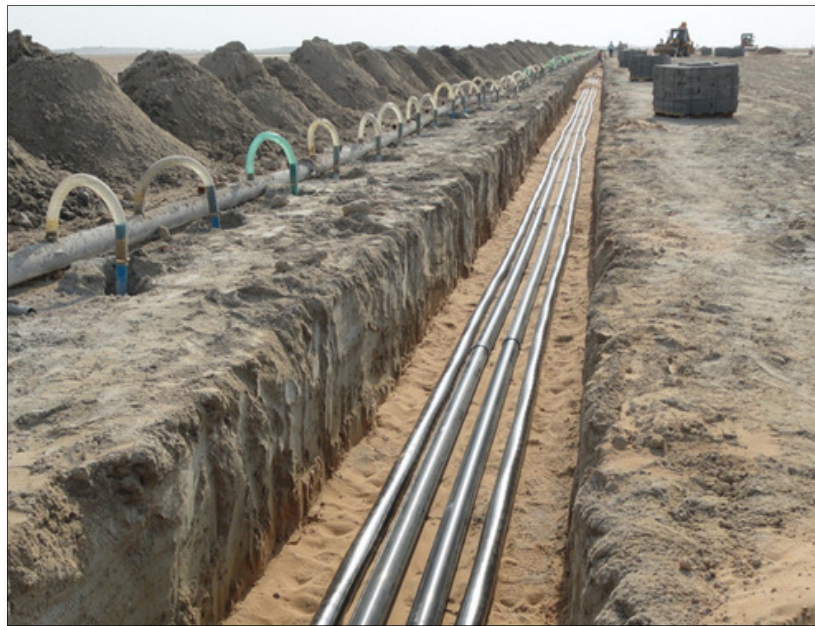
Figure (1) Underground Power Lines
