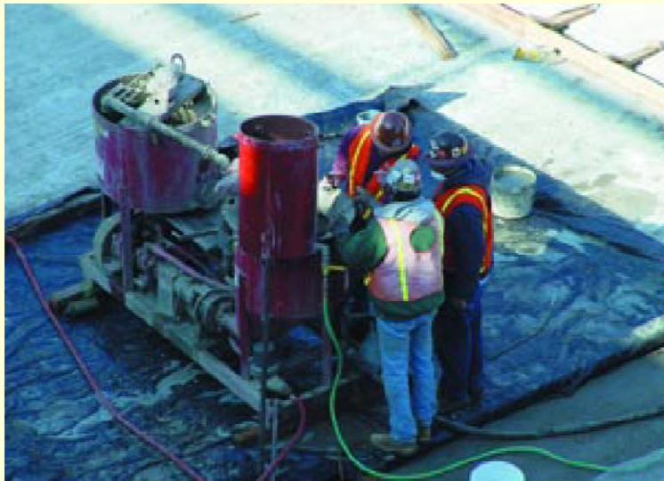
Mixing and pumping equipment
